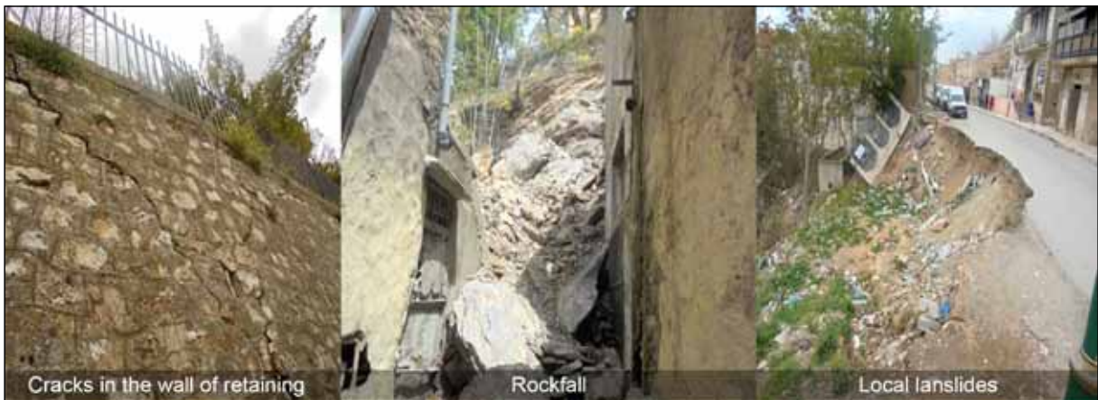
Figure 5. New instabilities registered in 2016.
