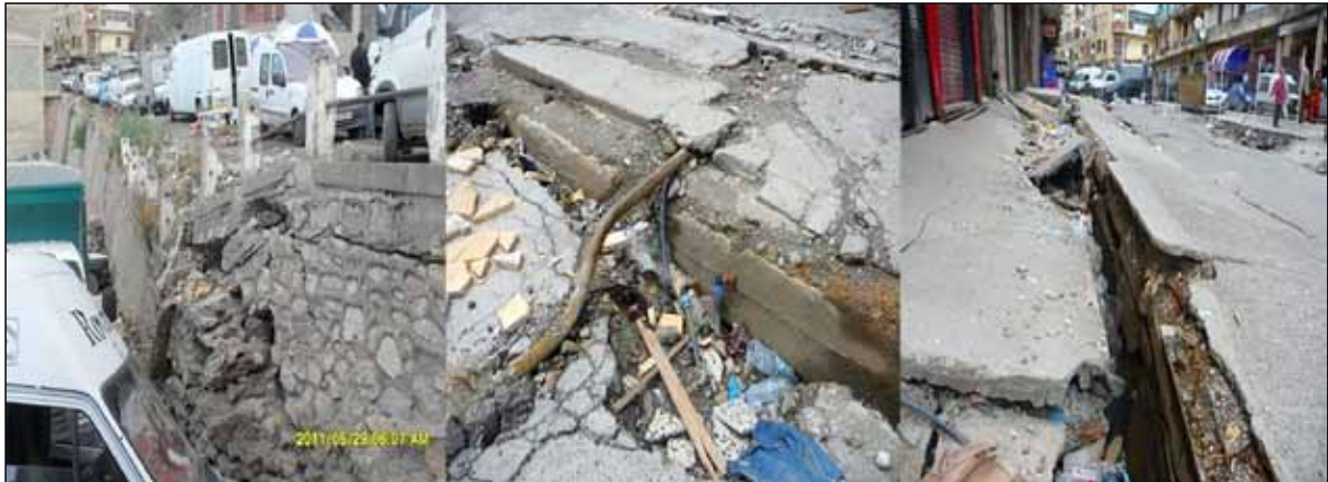
Figure 3. Dislocation of a retaining wall, subsidence of sidewalks, and cracks in pavements affecting pipeline networks.
