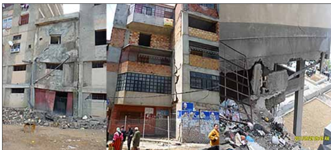
Figure 2. Obstructions observed in buildings.
