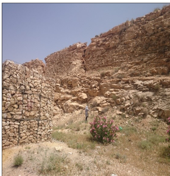
Figure 29. The active landslide along the highway in the Salhub area after cutting the foothill in station-6.
