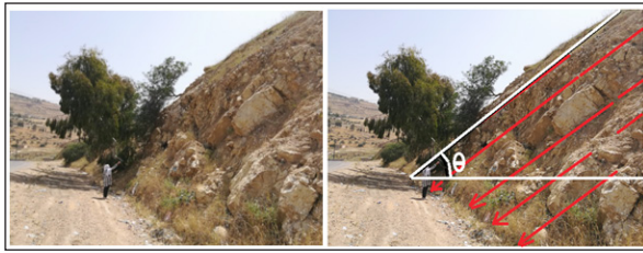
Figure 24. Plane sliding in station- 5.
