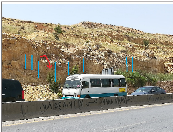
Figure 21. Vertically jointed Naur limestone cliff (blue lines) probable to topple in station-5
