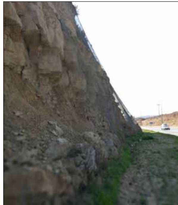
Figure 11. Shows wedge failure and the protruding overhanging rocks at the slope face.
