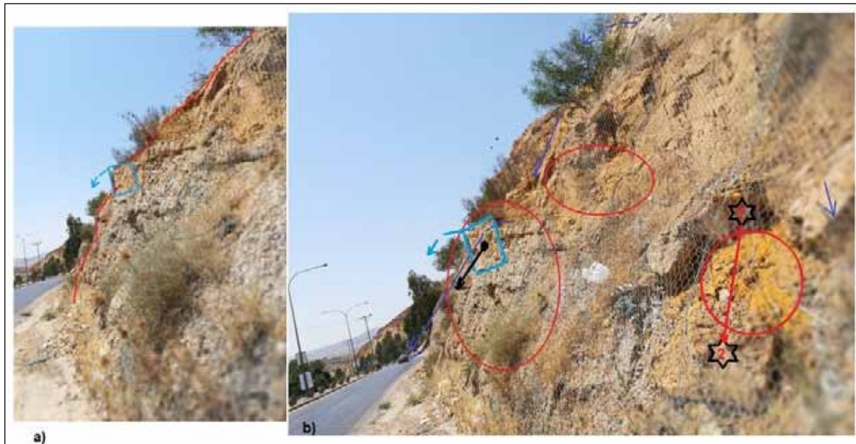
Figure 32. Side view of the Kurnub outcrop in station-7, it is yellow to dirty white, friable sandstone (red circle), highly weathered, and highly fractured (red ellipses). The block highlighted blue will topple, the black stars show the topple and slide the block from location 1 to 2.
