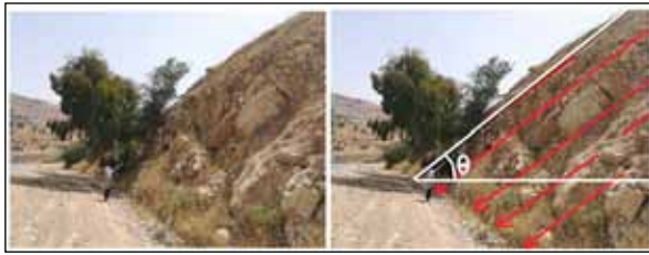
Figure 24. Plane sliding in station- 5.
