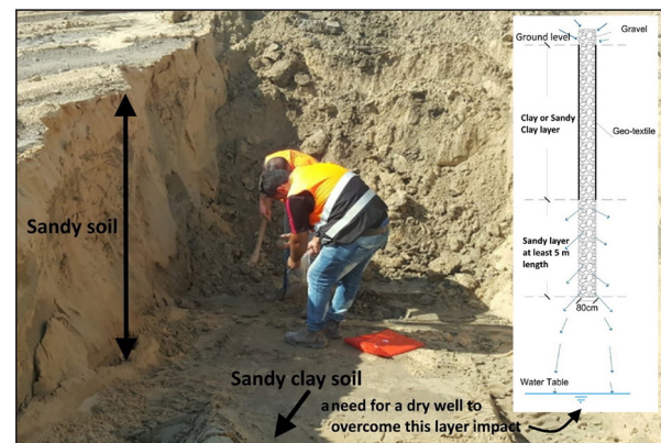
Figure 2. A real photo taken during the excavation for a stormwater pond depicting the need for dry well technique to penetrate a low permeable layer
