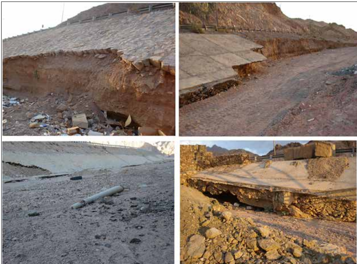
Figure 13. Undercut erosion at the base of the road
